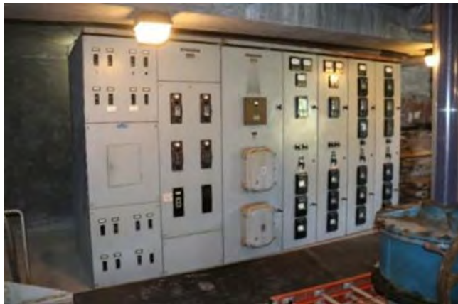
Shaft 5 - Electrical Switchgear to be replaced
