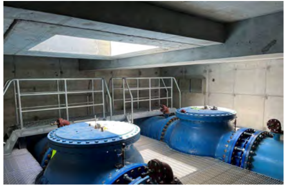
WASM 3 42-inch diameter PRVs
