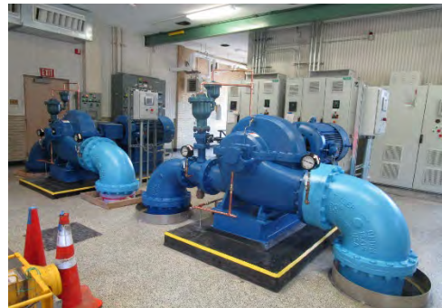
New Pumps at Commonwealth Avenue
